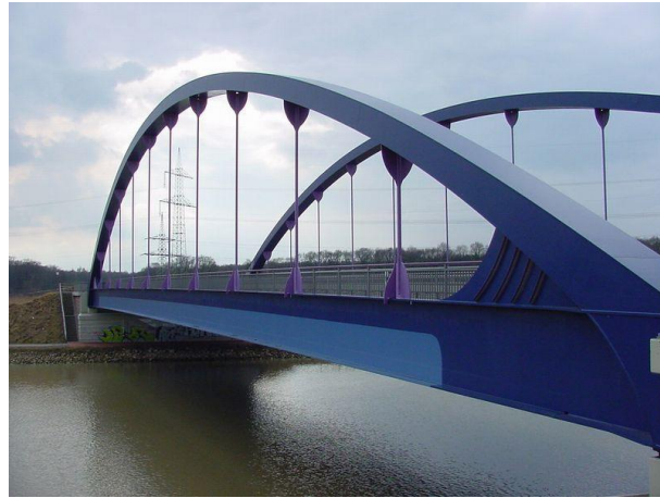
Figure 2.3: A bridge as representative of a man-made dynamic structure. Even if it appears static at first glance, the continuous care in terms of inspection and maintenance (interaction with the environment) should be kept in mind that is needed to retain its functionality over a long period of time.
