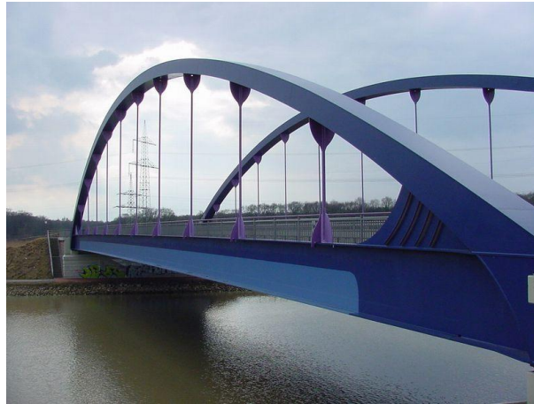
Abb. 5. A bridge as representative of a man-made dynamic structure. Even if it appears static at first glance, the continuous care in terms of inspection and maintenance should be kept in mind that is needed to retain its functionality over a long period of time.
